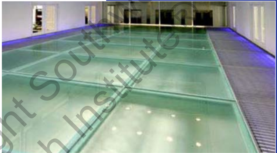
SwRI listed and labeled floor/ceiling assembly
