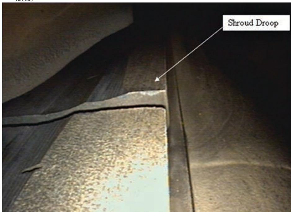
The shroud droop and damaged turbine blades are shown in the borescope images from the maintenance inspection.
